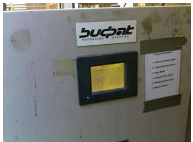
EQUIPMENT CONTROL PANEL
