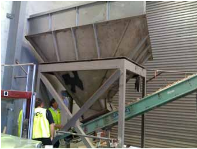
LOADING HOPPER WITH INCLINED PRODUCT TRANSFER CONVEYOR
