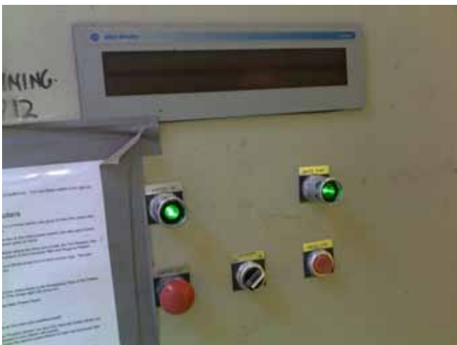
EQUIPMENT CONTROL PANEL
